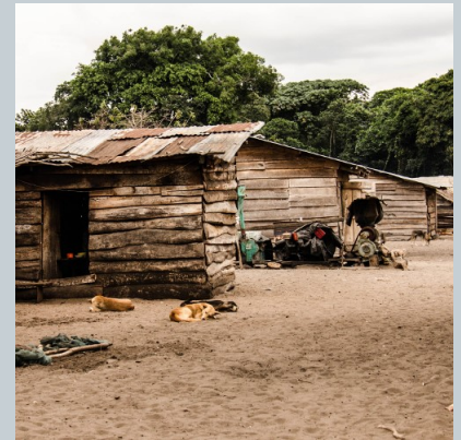
Unsafe housing in nearby community.
